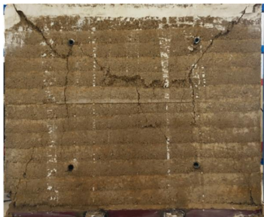
Fig. 15. Crack Pattern from experiment [6].
